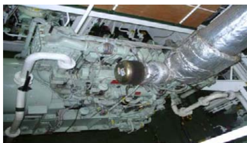
Generator engine 530kw 1,200min -1 3sets
