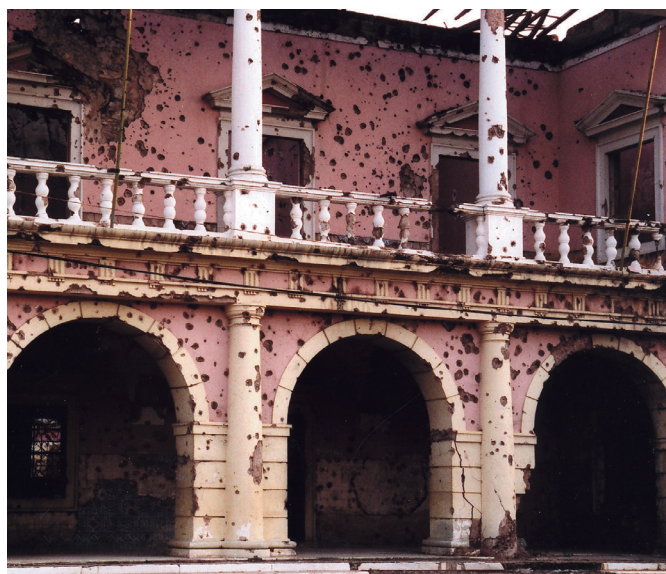
Many public buildings lay in ruins in the aftermath of Angola's civil war. (Kuito City, Bie Province)
